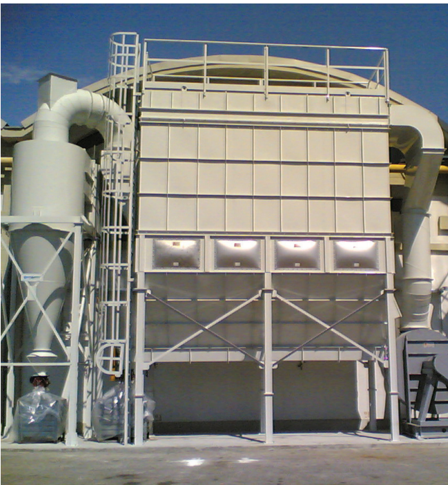
■ Dust extraction and filtration system for powders from mechanical processing - Italy
