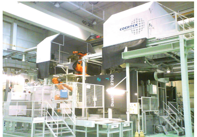
■ Hood into two parts on FRECH DUALCAST 2700 die-casting machine connected to a centralized suction and filtration system ENERPROG
