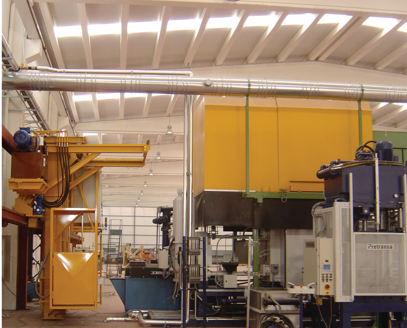
■ Automatic ladle wagon for the pouring of aluminum into holding furnaces at the service of die-casting machines - Spain
