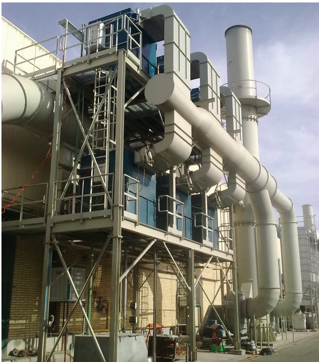
ENERPROG centralized intake and filtration system in 6 modules dedicated to 4 large tonnage presses - Iran
