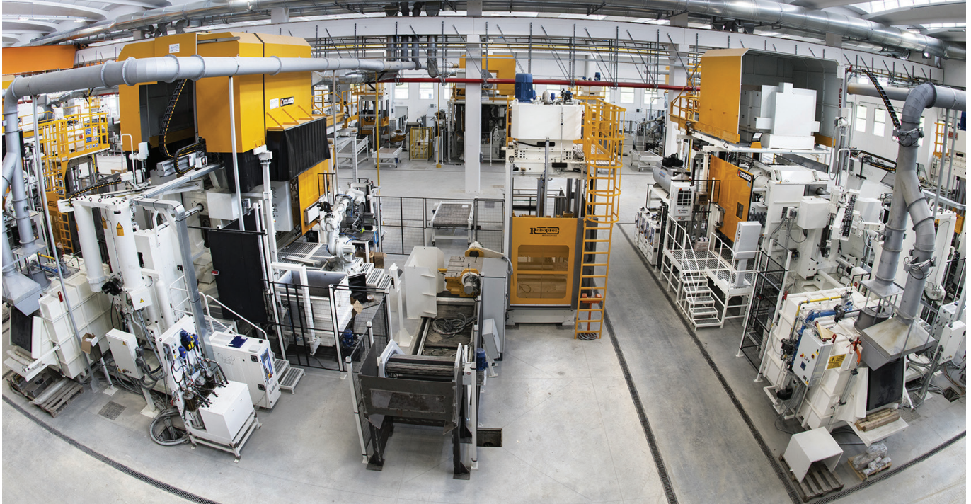
Two parts hoods on die casting machines complete with ENERORESS filters, extraction fans and expulsion chimneys - Italy
