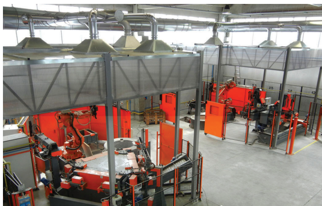
■ Extraction hoods on gravity casting cells connected to a centralized suction and filtration system - Italy
