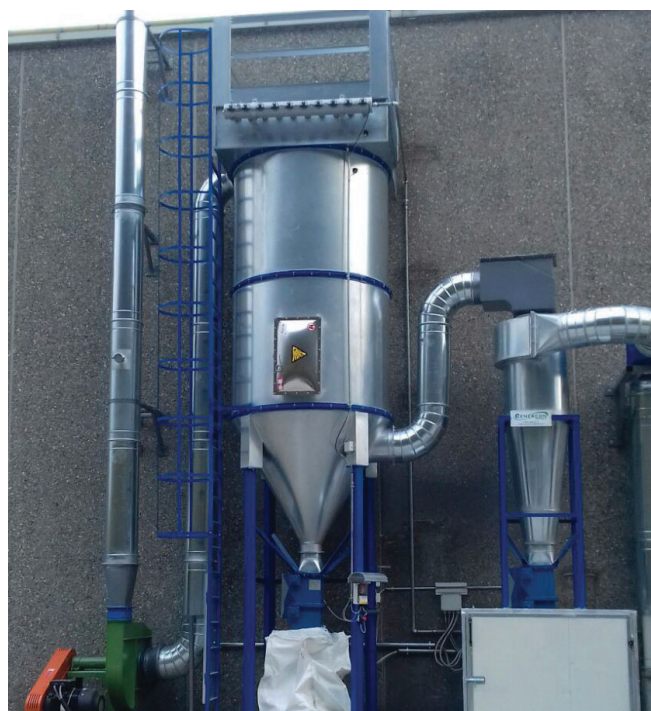
■ Suction and filtration system from aluminum cutting powders -6.000 m³/h
