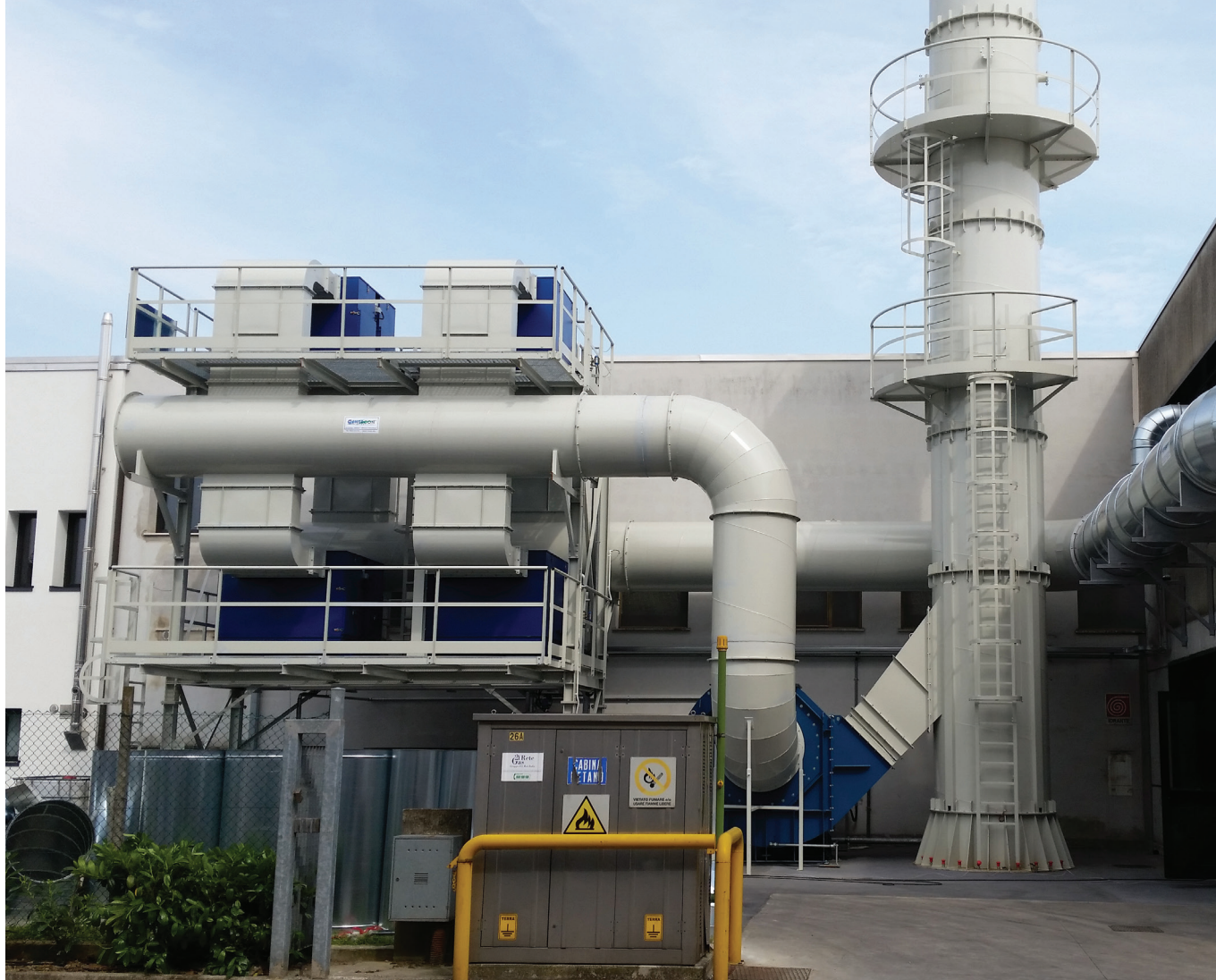
ENERPROG centralized suction and filtration system in 4 modules dedicated to 7 presses - Italy
