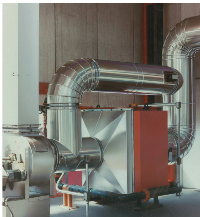
■ Fume/water heat exchanger for the use of heated water inside the plant - Italy
