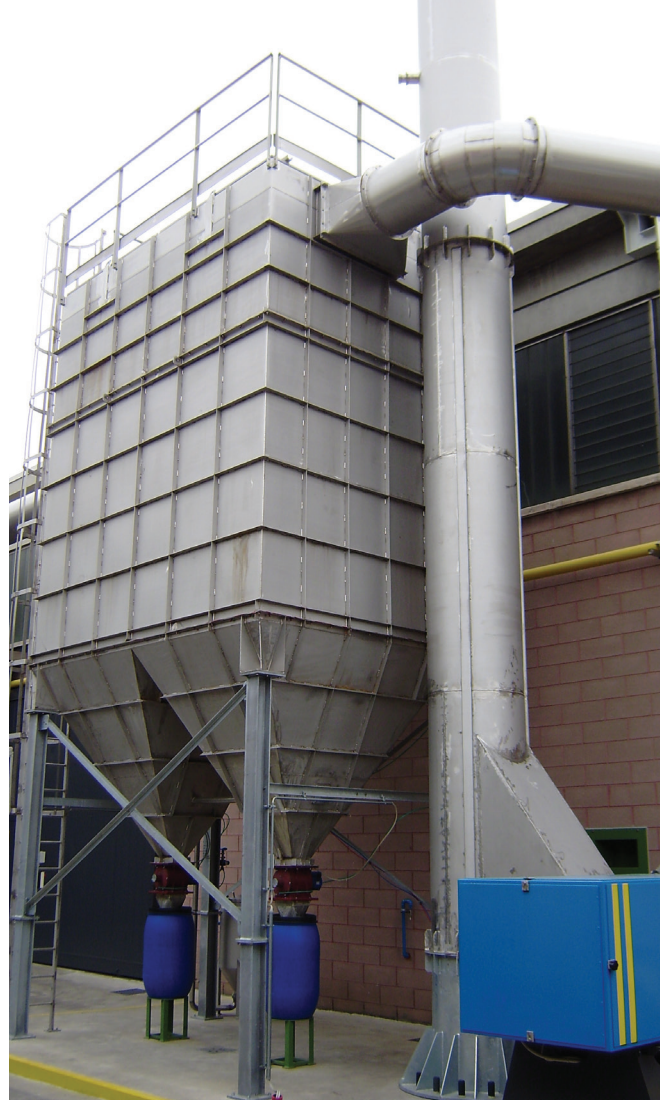
■ Suction and filtration system for bronze dusts - Italy
