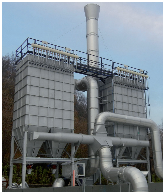
■ Suction and filtration system for fumes from furnaces. Italy
