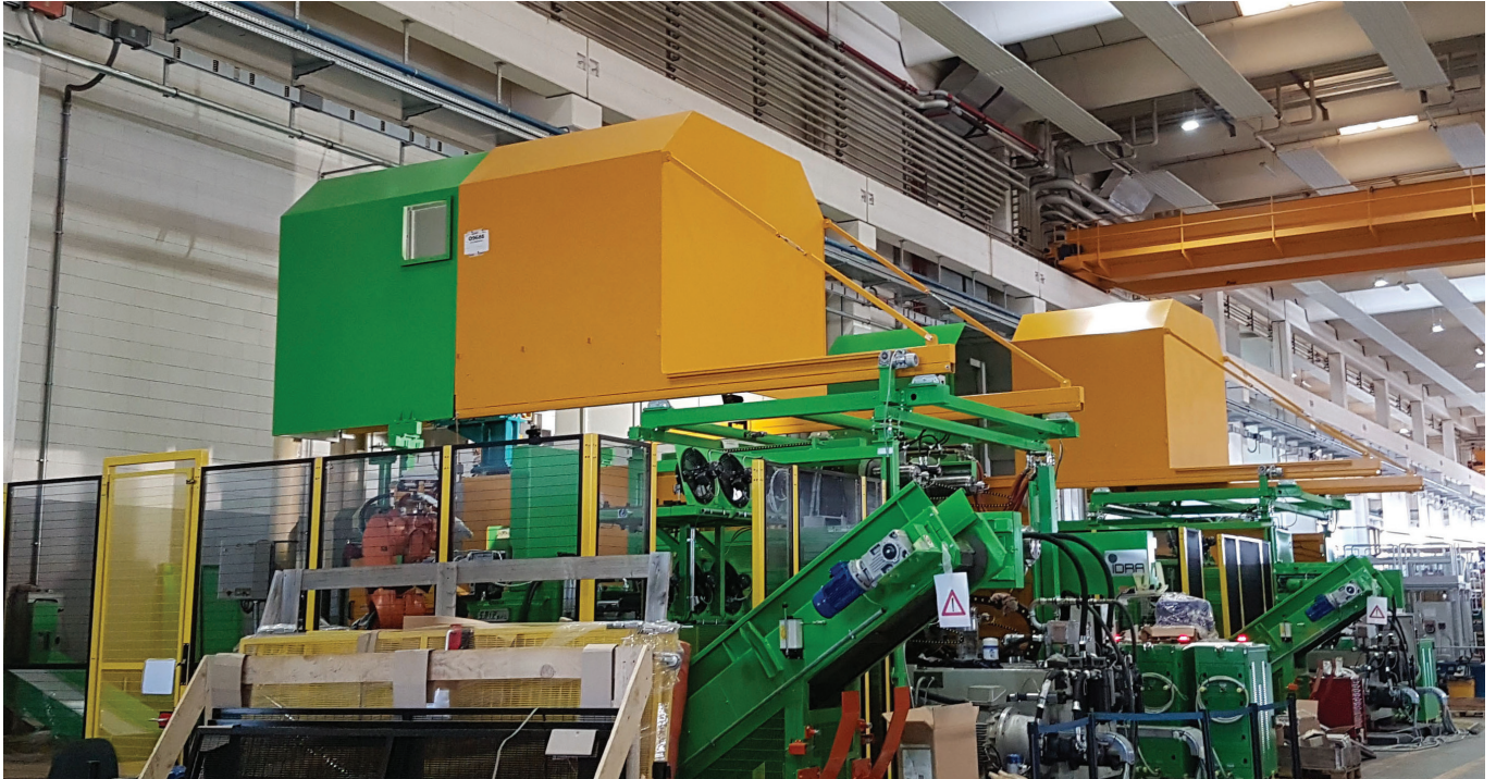
■ Hoods on presses connected to a centralized suction and filtration system - Uzbekistan
