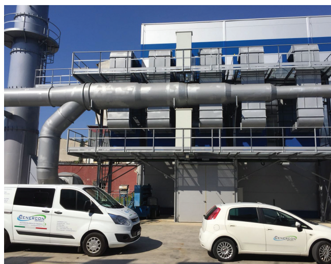
ENERPROG centralized suction and filtration system in 10 modules for a total suctioned flow of 150,000 m 3 /h for 19 presses - Slovakia
