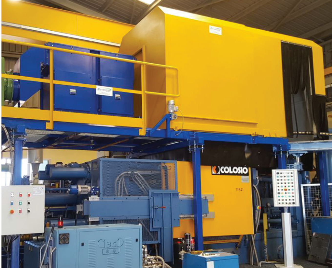
■ Hood into two parts complete with individual ENERPRESS filtration system, fan and individual chimney for the expulsion in the atmosphere of purified air on COLOSIO PFO560 die-casting machine - Spain
