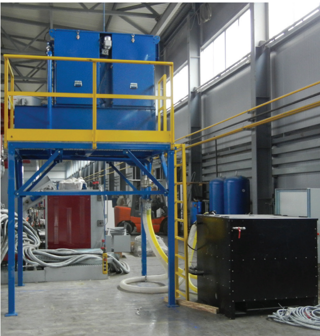
ENERPRESS filter on an independent structure with mobile washing tank beside it, dedicated to a single die-casting machine and connected to a centralized suction unit. Ukraine
