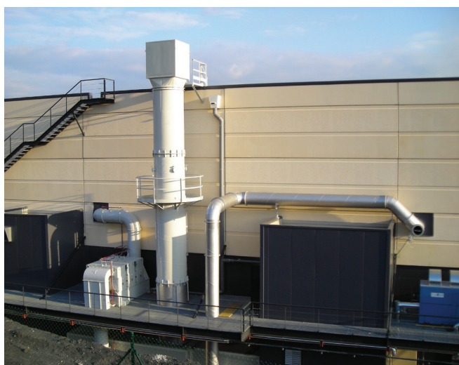
ENERPROG centralized suction and filtration system in number 2 modules for a total sucked flow of 32,000 m 3 /h dedicated to 4 presses - Spain
