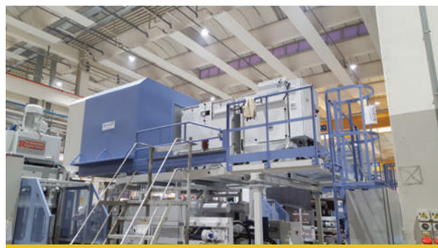
Hood into two parts complete with individual ENERPRESS suction and filtration system for recirculation of purified air in an environment on IDRA OL420S die-casting machine – Poland
