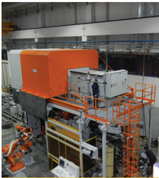
Hood into two parts complete with individual ENERPRESS suction and filtration system for recirculation of purified air in a die-casting machine – Russia
