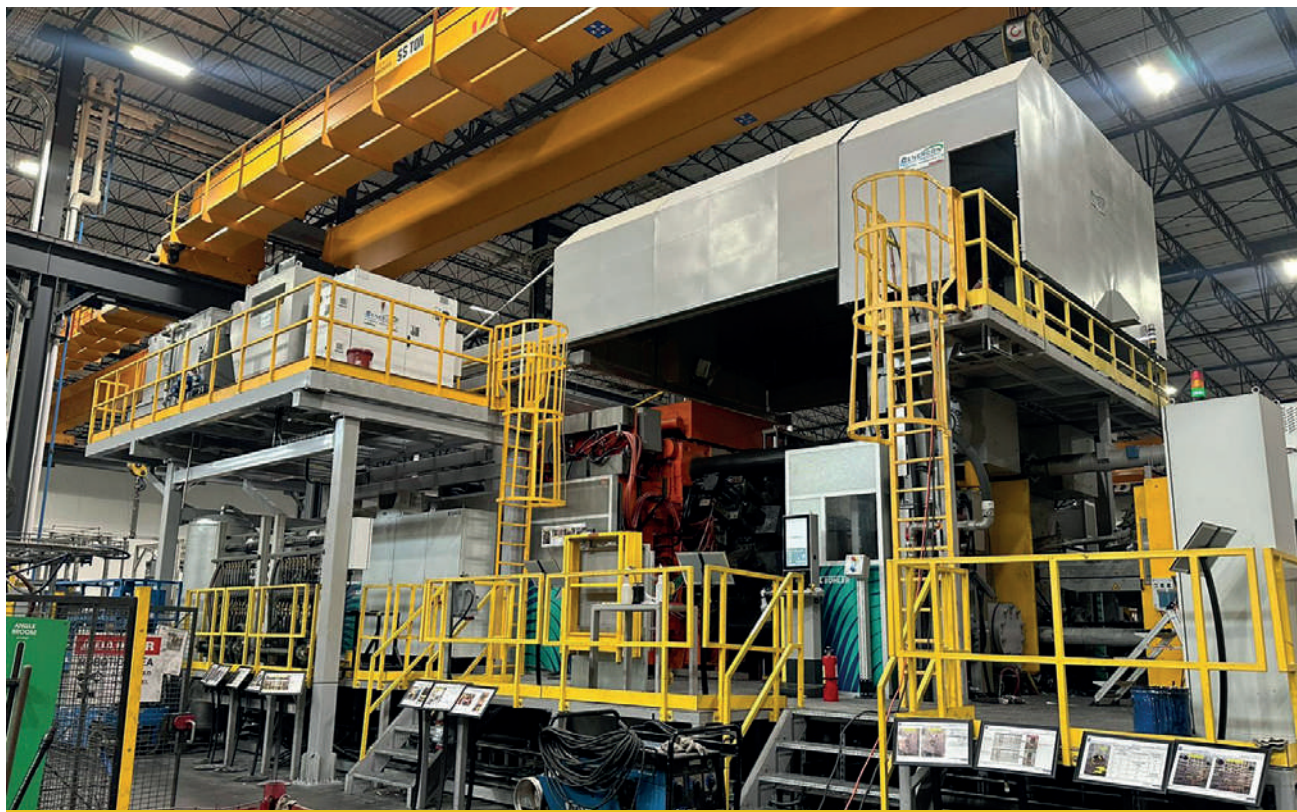
Hood on a 4500 Ton die-casting machine complete with self-cleaning ENERPRESS electrostatic filter for recirculation of purified air into the workplace, installed on an independent platform – USA
