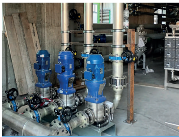
Lifting station with in-line pumps in water treatment plant – Italy
