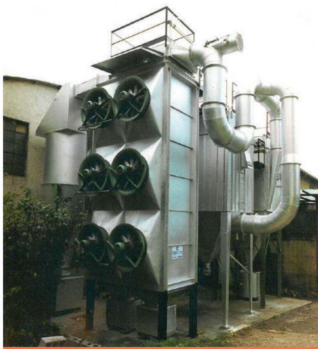
■ Examples of fume/air heat exchangers installed on aspirations from melting furnaces complete with insertion of the heated air inside the production departments with high energy recovery.
