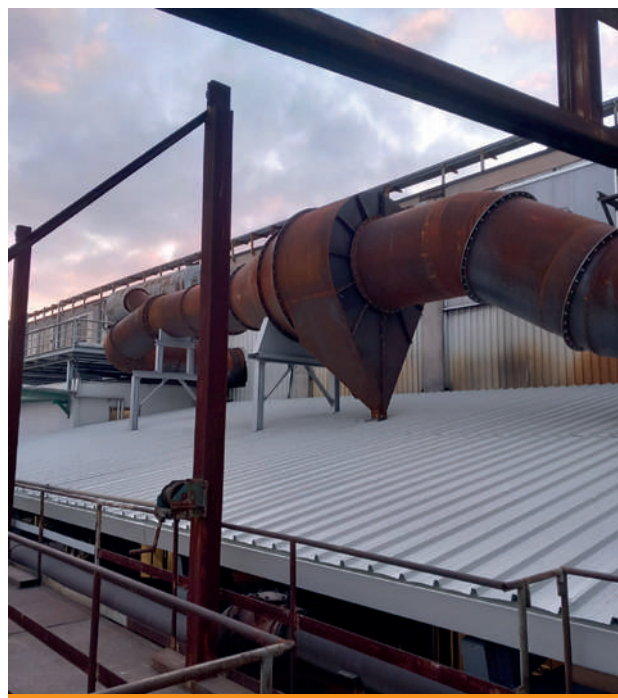
Axial cyclone for coarse dust abatement and spark arresting in aspiration and filtration plant – Italy
