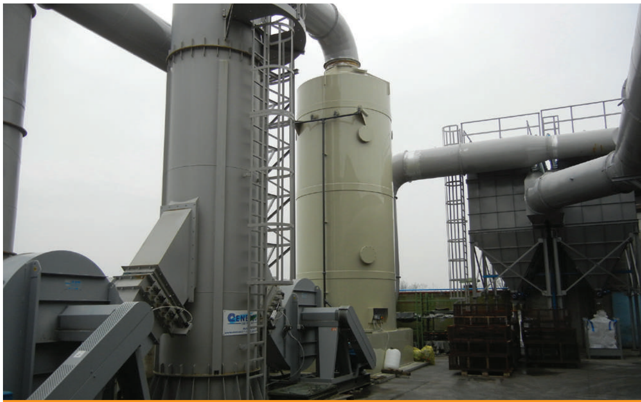
Technological systems for suction, dust filtration and odor abatement from bronze shell casting machines and bronze melting furnaces – Italy
