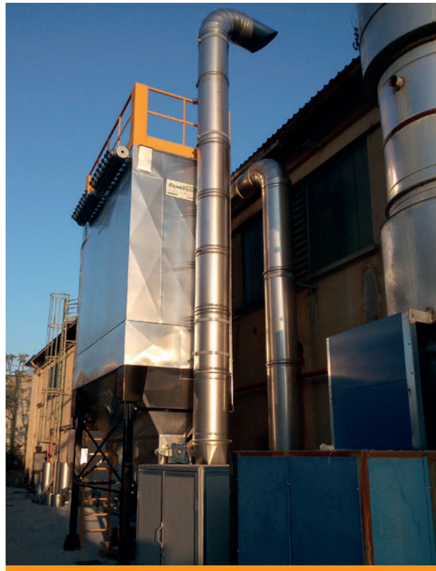
Aspiration and filtration plant for aluminium tower melting furnace – Italy
