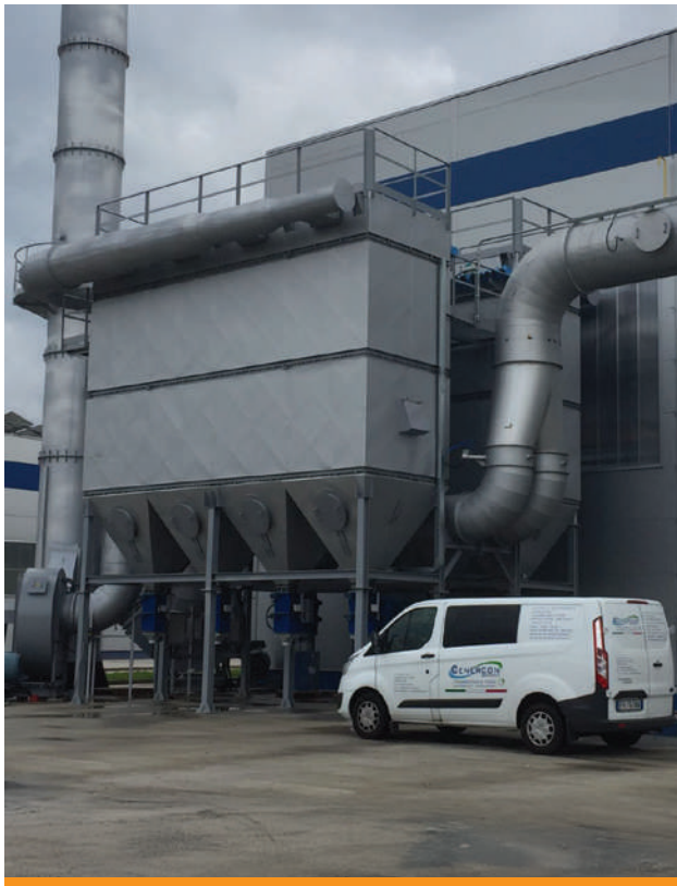
85,000 m 3 /h suction and filtration system for fumes treatment from aluminum melting furnaces – Slovakia
