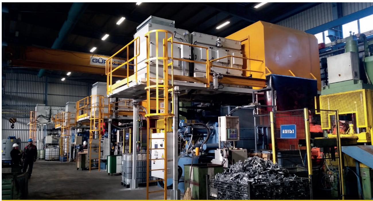
Hoods on die-casting machines complete with self-cleaning ENERPRESS electrostatic filters for recirculation of purified air into the workplace – Turkey
