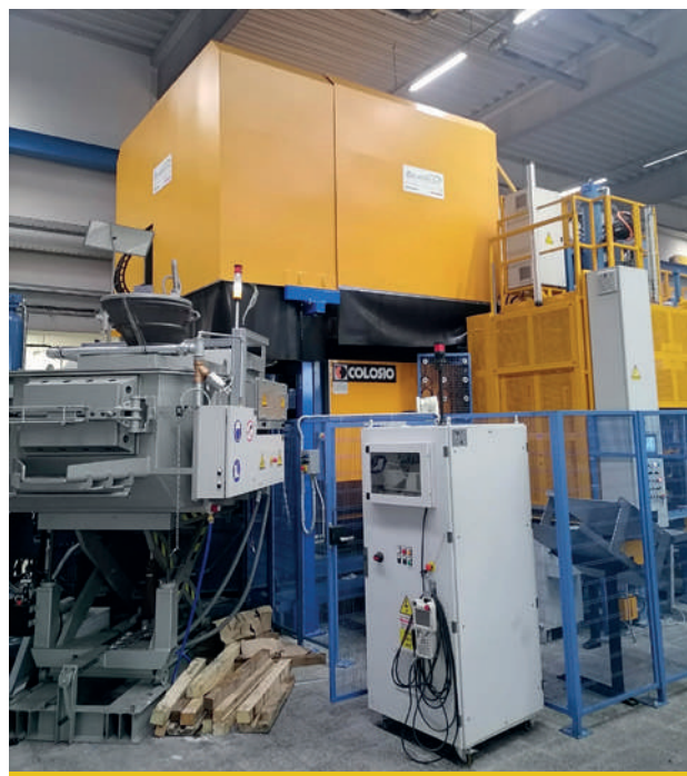
Hood on a 750 Ton die-casting machine complete with self-cleaning ENERPRESS electrostatic filter for recirculation of purified air into the workplace – Czech Republic
