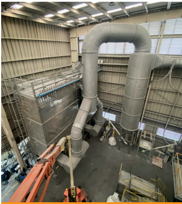
Aspiration and filtration plant for fumes from 3 aluminium melting furnaces, 1 dryer and 2 degassing stations, capacity 100,000 m 3 /h, complete with inertisation system for acidic pollutants – Mexico
