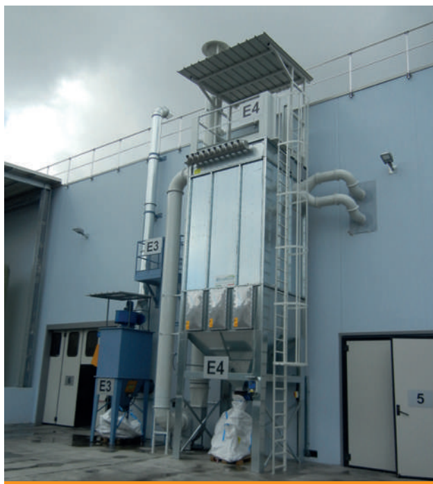
Aspiration and filtration plant for aluminium dust from manual grinding – Italy
