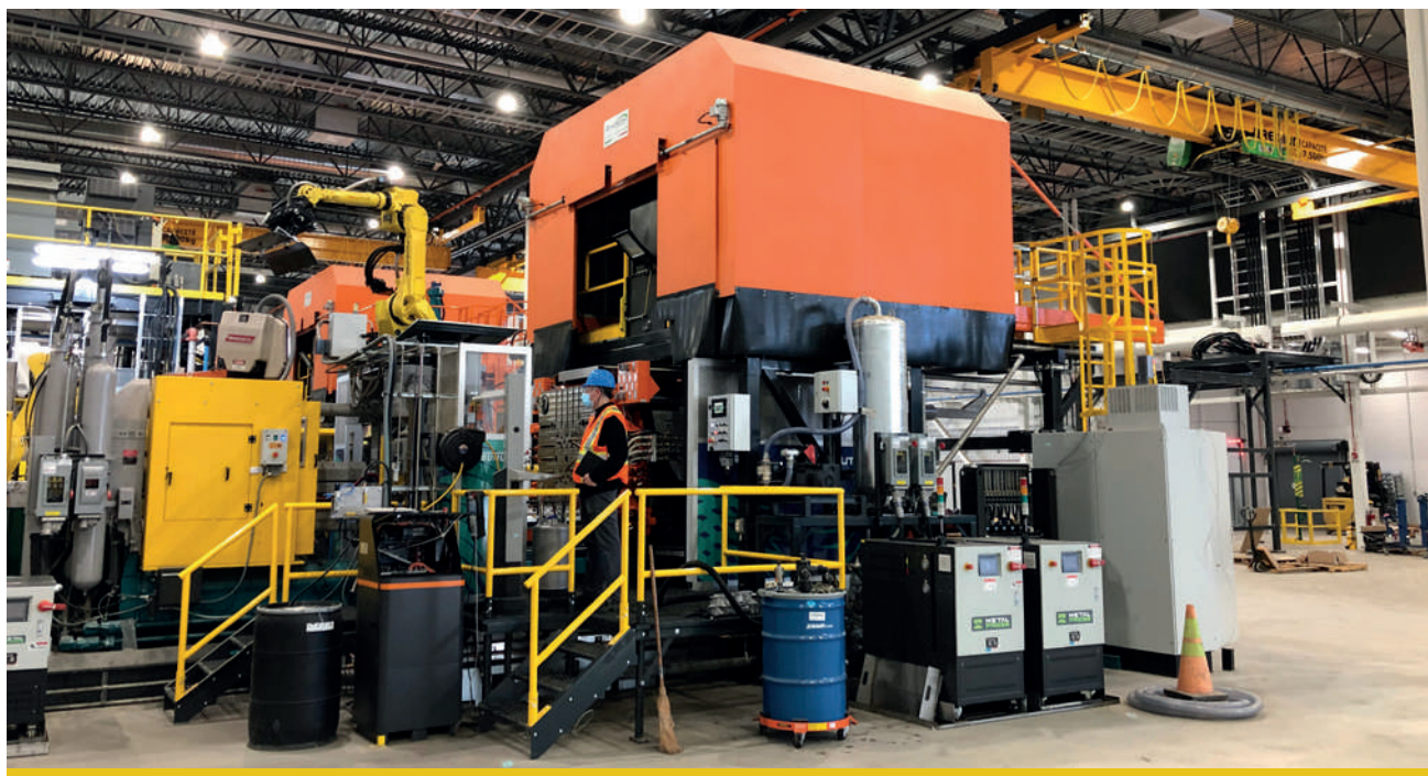
One-piece hoods with automatic opening door for lubricator passage, on die-casting machines from 600 to 1400 Ton, complete with self-cleaning ENERPRESS electrostatic filters for recirculation of purified air into the workplace – Canada
