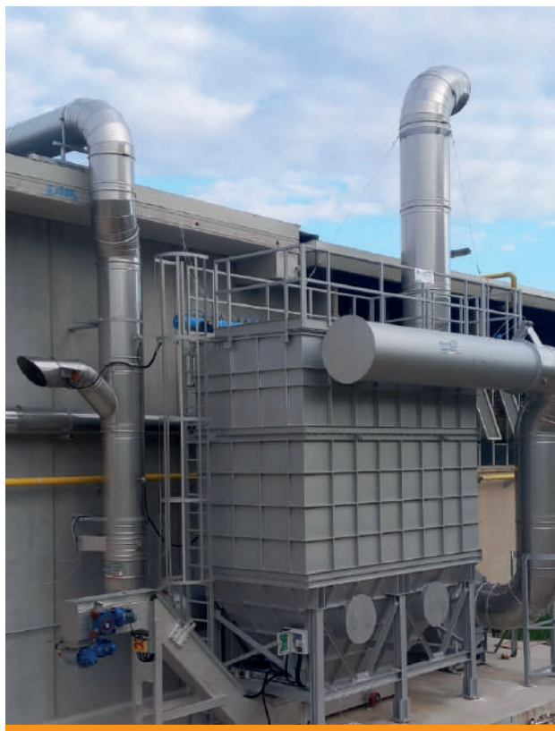
■ Dust aspiration and filtration plant with lowered discharge and Redler dust transport system – Italy
