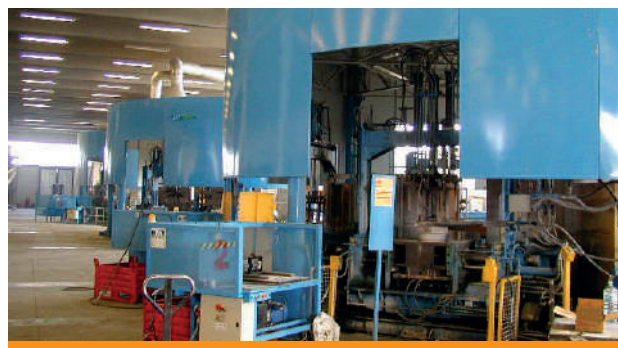
■ Aspiration hoods on shell moulding machines connected to a centralised aspiration and filtration plant – Italy
