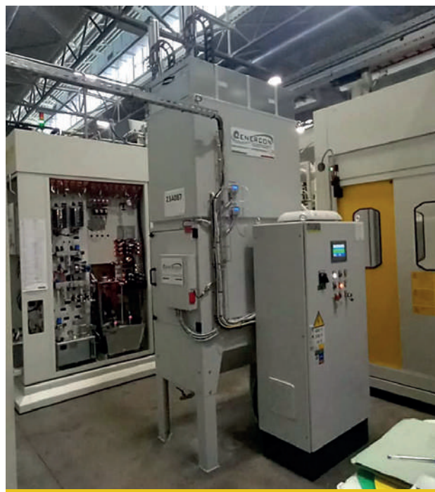
Aspiration and electrostatic filtration system for recirculation of purified air from 4 machining centres. Czech Republic
