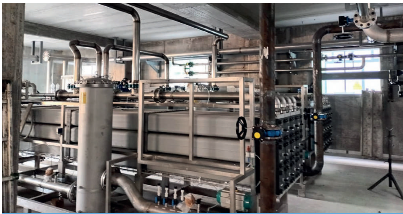
Reverse osmosis plant for purification of industrial water. Compact skid-mounted structure with high-efficiency membranes. Italy
